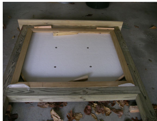
Photo 2-6: Homosote screwed in place. Window frame in position supported by spacer scraps.
